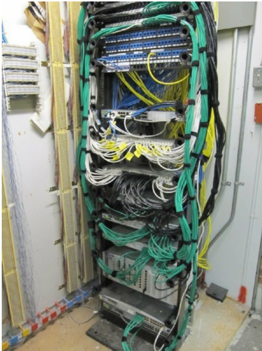
Figure 10.1 A typical wiring closet
